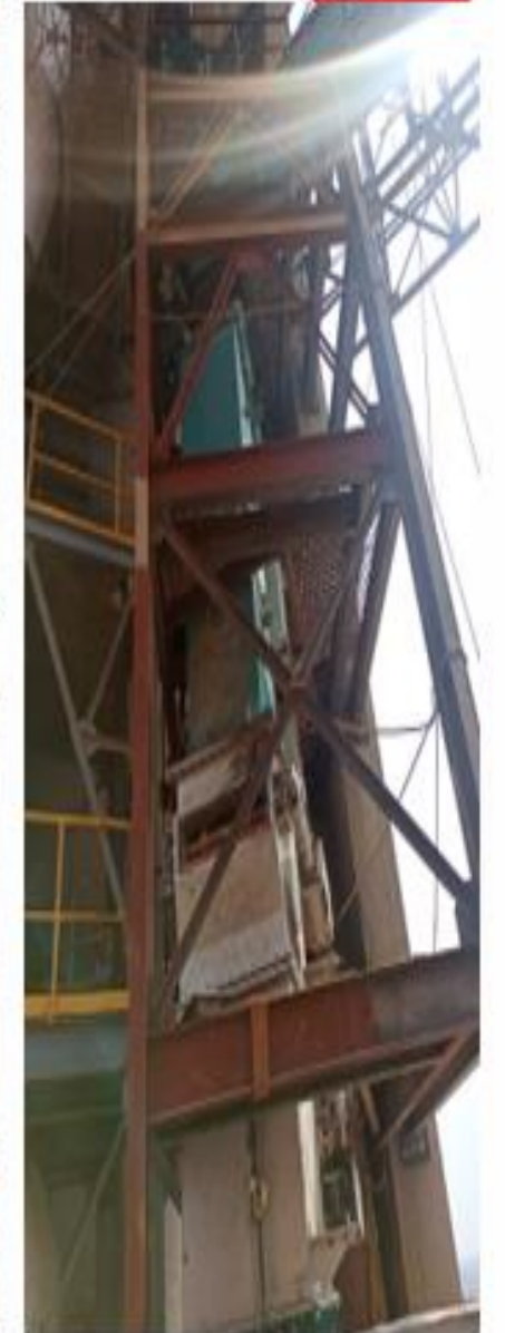
Feeding System at Preheater
